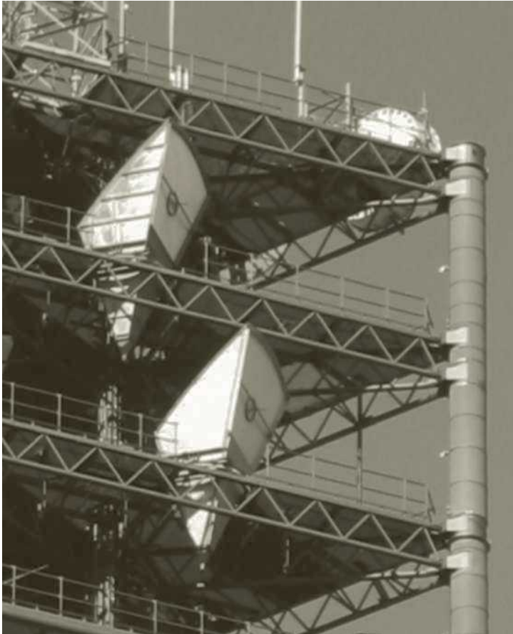
Figure 4-14 Telephone transmission tower showing two horn antennas
