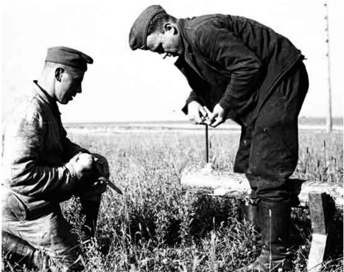
Top and above: ...before they are screwed into telephone poles to support the bare wire cables.
