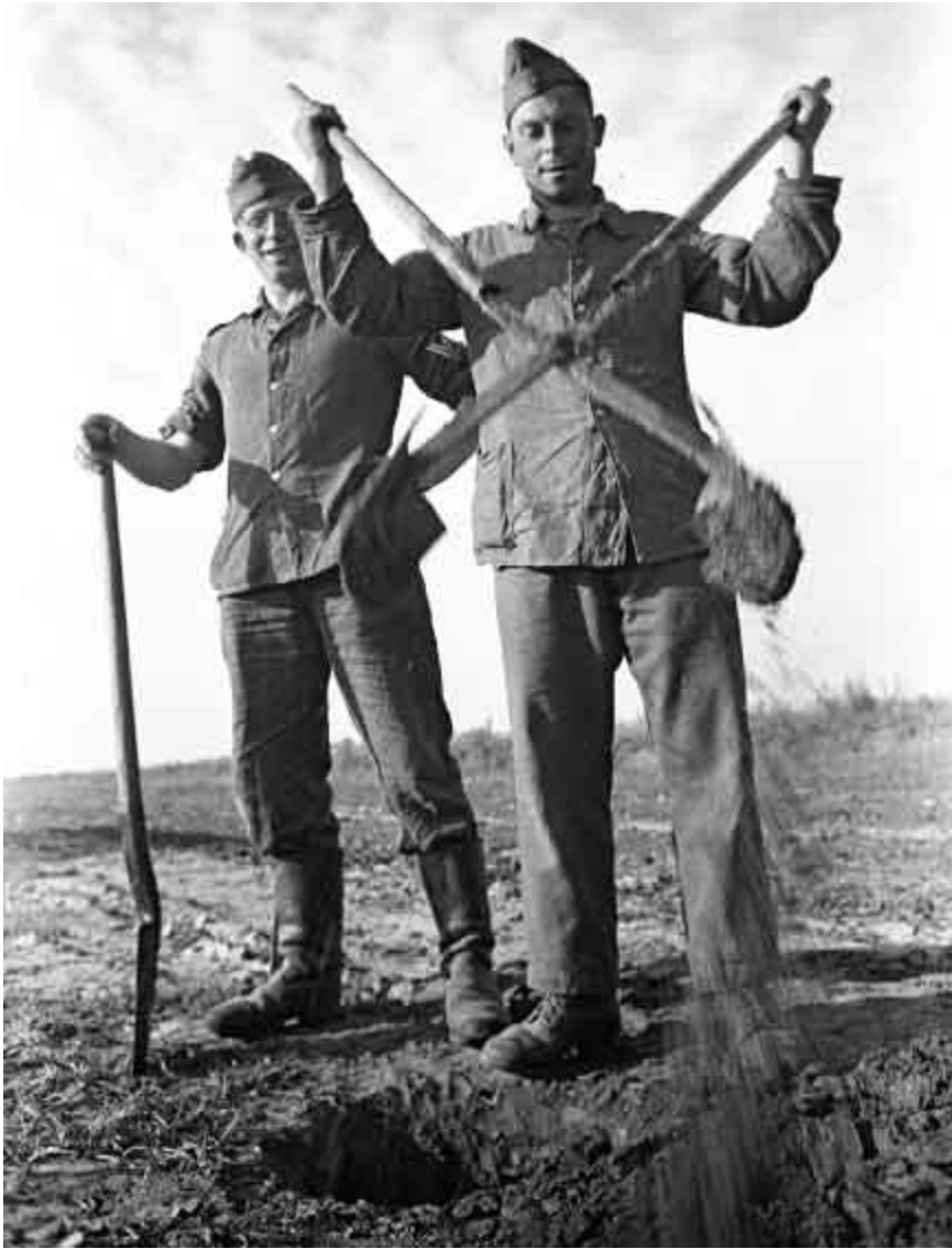
Top and above: Digging holes for telegraph poles using a tool known in German as a Doppelspaten (double spade) or Lochspaten (hole spade).
