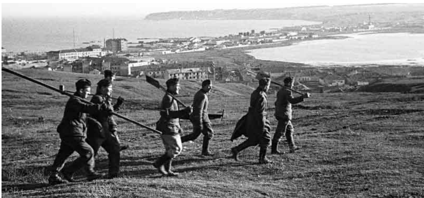
Top and above: Erection of Drehkreuz lines in Crimea; the Black Sea is visible in the background. The men wear the dark green Drillichrock tunic.
